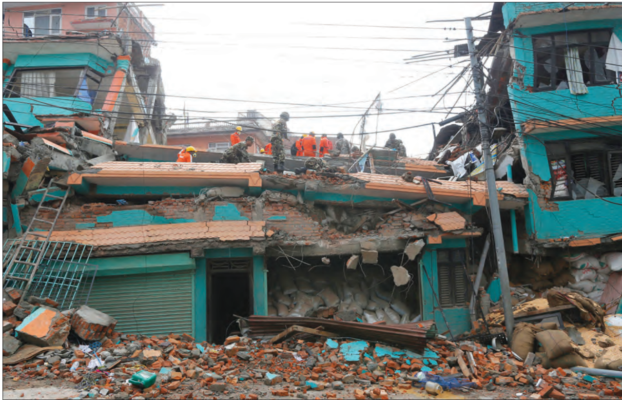
Rescue teams search for bodies on Monday in the collapsed Sitapyla church in Kathmandu, Nepal. A strong earthquake shook Nepal's capital and the densely populated Kathmandu Valley on Saturday. The catastrophe has overwhelmed Nepal's government, with the challenge expected to worsen as the death toll climbs. Four thousand people were confirmed dead Monday.
